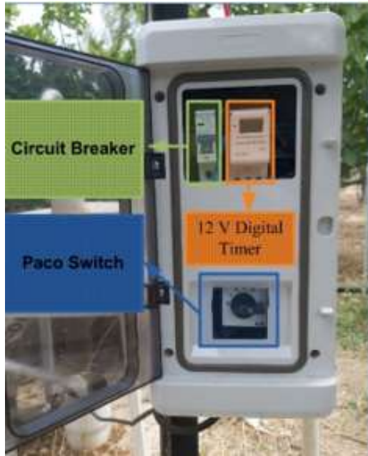
Figure 6. Control unit of solar water pumping system in use
