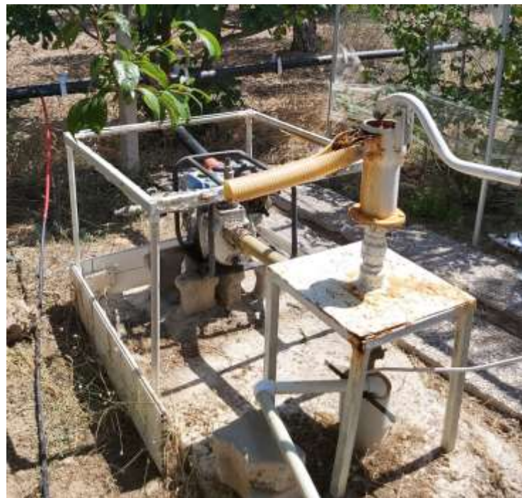
Figure 5. Photograph of the gasoline-based water pumping system in use
