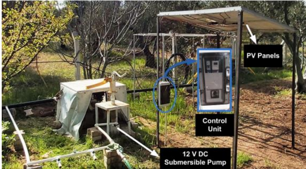
Figure 5. Photograph of the solar water pumping system in use
